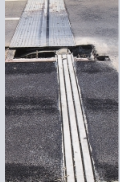
Replacement of a Roller Leaf Joint by a MAURER Swivel Joist Expansion Joint
